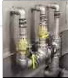
Stainless steel moisture blow-off header pipers with control valves.
