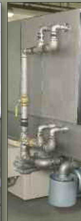
Moisture blow-off header pipes for both above and below belt coverage of heated air.
