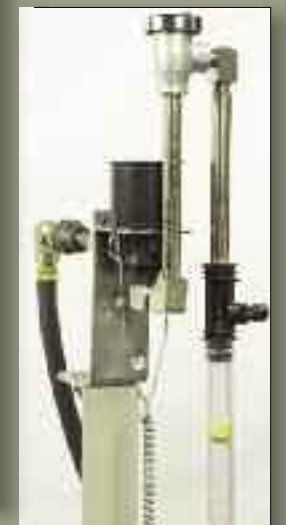
Cleaning chemical automatic make-up system.
