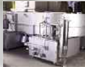
#1 rinse station showing hood and stainless steel bag filtration system.
