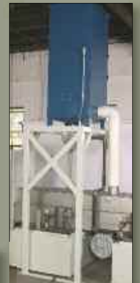
Mist collector complete with Almco manufactured frame work and exhaust ducting.
